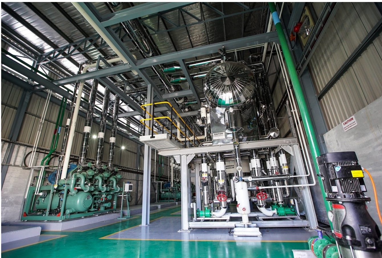
CaaS ammonia refrigeration system at a poultry producing plant of Sovereign Foods, South Africa
