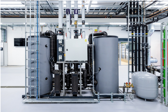
CO 2 Refrigeration & Heat Recovery Special Edition
